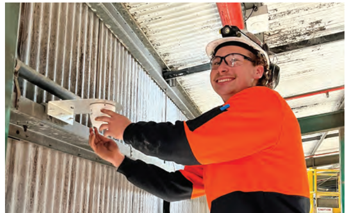
Cameras were installed at the sorter by Electrical Apprentice, Tanner Fratantaro.
