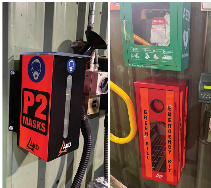
P2 Dust Mask Dispenser and Emergency Go Kits have been installed.
